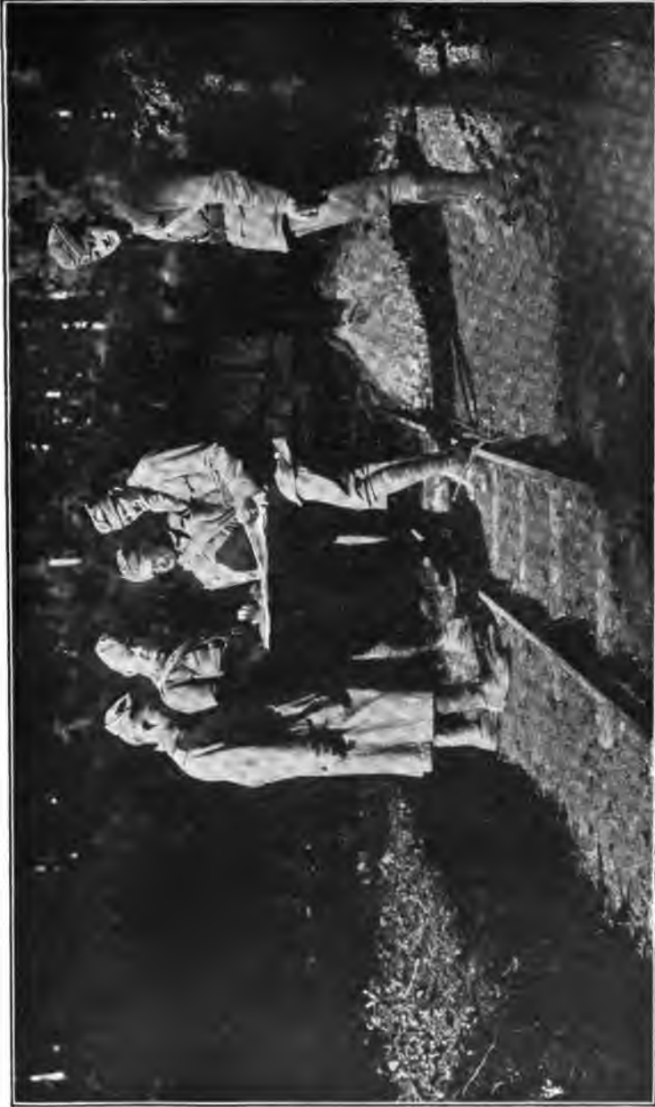
AMERICAN ENGINEERS CONSTRUCTING A LIGHT RAILWAY THROUGH A FOREST WHERE IT COULD NOT BE DISCOVERED BY ENEMY AIR OBSERVERS
